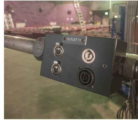
▲ Custom made power and DMX outlet
