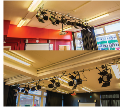
▲ Classroom Lighting Installations
