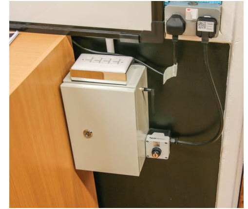
▲ Lighting Control Box with Scene Select Switches
